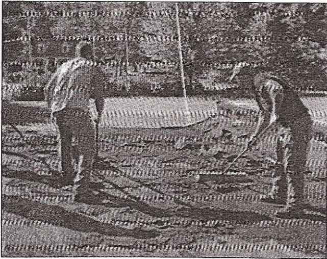
Workers from NorthStar Construction Services Corp. help replace the roof at Saima Park. The company donated time and $2,000 in materials to fix the roof.
